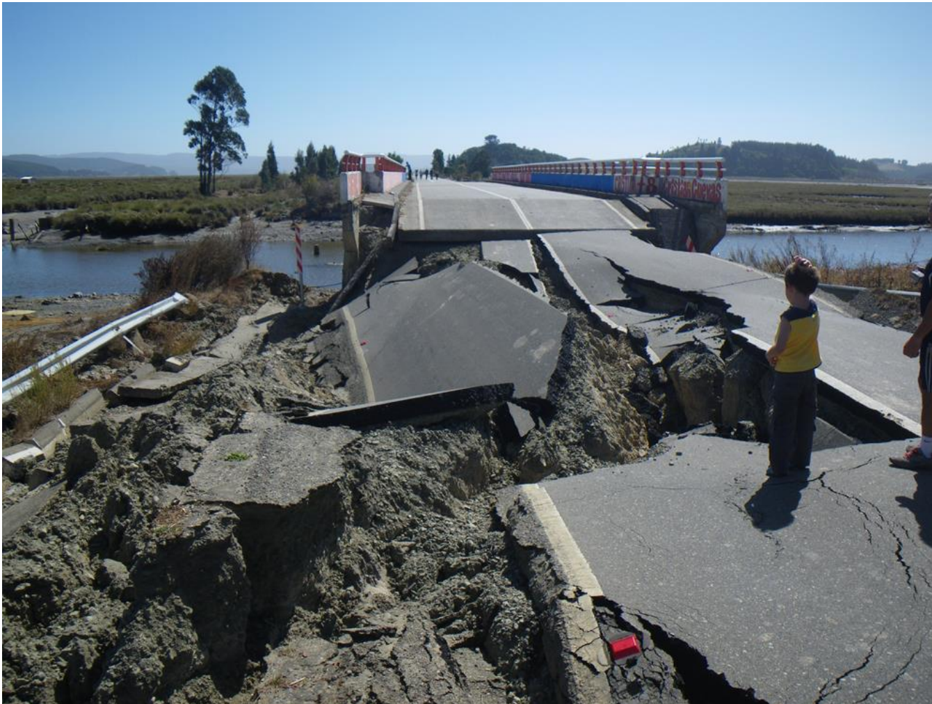
Shaking damage in the Arauco Peninsula, south of Concepción
